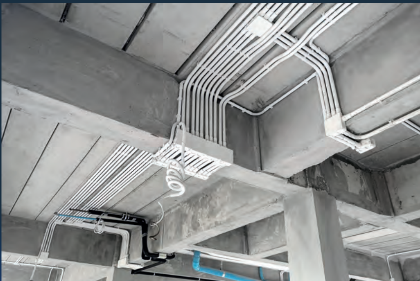
INFRASTRUCTURE CEILING - ELECTRICAL CONDUITS
