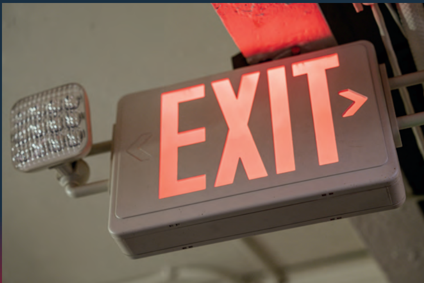
OFFICE COMPLEX PARKING - LED COMBO LIGHT
